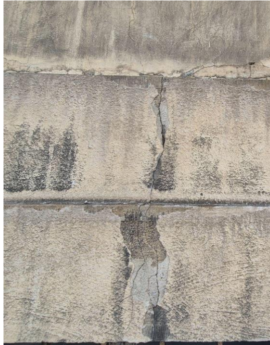
Lower part of front facade: Remove cement render, repair historic lime plaster, and restore missing decorative elements.
